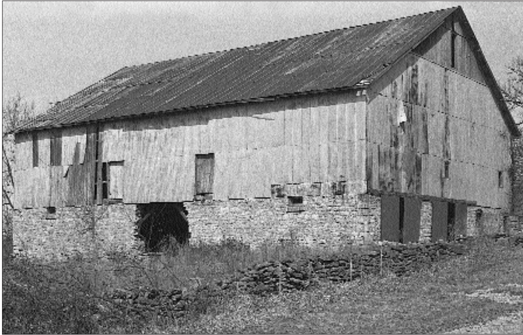
Fig. 12: In later years a hole unfortunately was punched in the limestone foundation on the south barn-yard side of the Henry barn.
